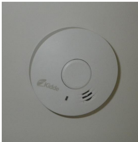
Rookmelder in appartement
