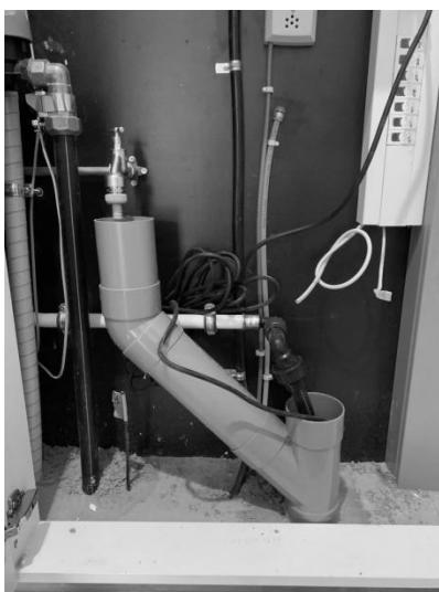
Regenwaterinstallatie in nis in inkom
