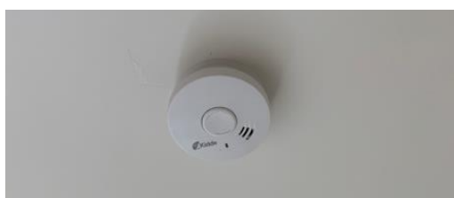
Rookmelder in appartement
