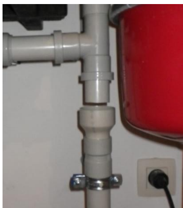
Vrije overloop regenwaterpomp
