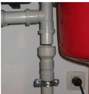
Vrije overloop regenwaterpomp
