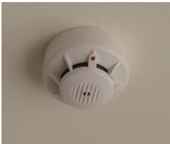
Rookmelder in woning
