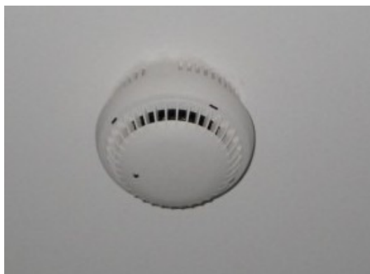
Rookmelder in appartement
