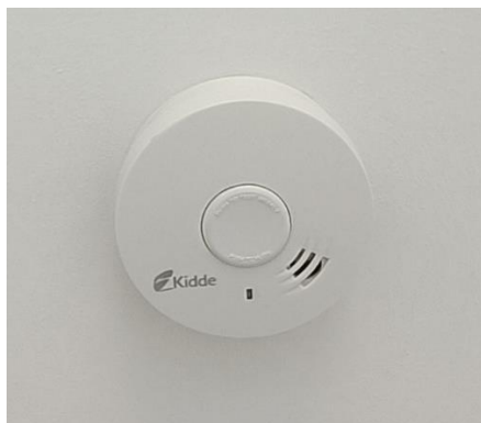
Rookmelder in appartement
