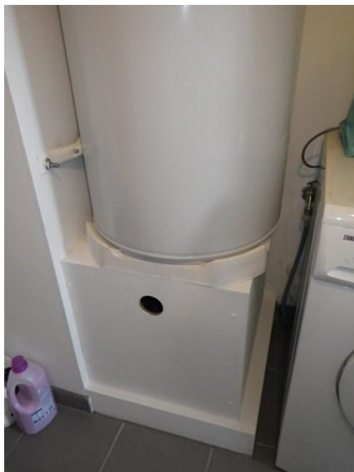
Boiler met controleopening
